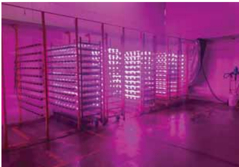
Figure 1. The enhanced rooting chamber at Battlefield Farms, Virginia. Shipping carts of young plants are lit by LEDs mounted horizontally in bays.
